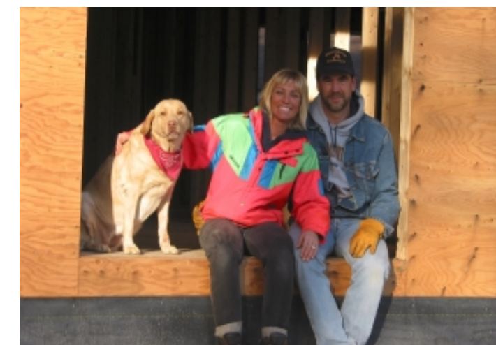
This opening where Mike and LuAnn are sitting will soon become a patio door located in their master bedroom. It will allow them to walk out to a deck that spans the rear of the house.
